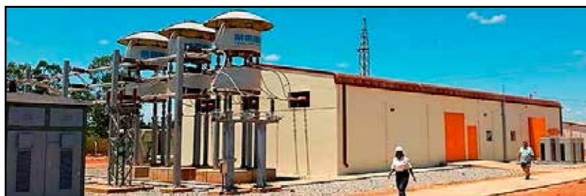
Figure 2: ± 75MVAR, 220kV STATCOM System inside civil building (Courtesy: Montnets Rongxin Technology Group Co., Ltd)
